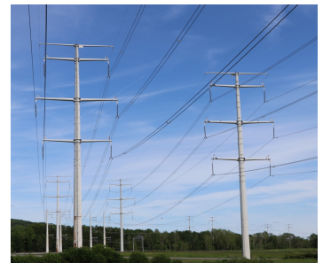
Figure 1.1 345,000 volt transmission lines.
