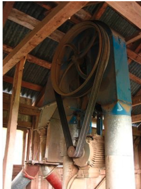
(b) Power transmission pulleys.
